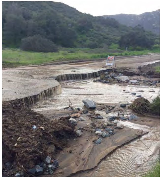
Lilac Road crosses a natural flood plain and is vulnerable to overflow from Bubble Up Creek and the San Luis Rey River
