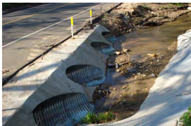
Culverts on Pala Creek passing under Pala Temecula Road are vulnerable to clogging during every rainstorm, causing flooding that makes the road impassable
